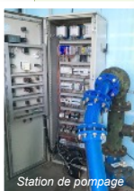
Station de pompage
